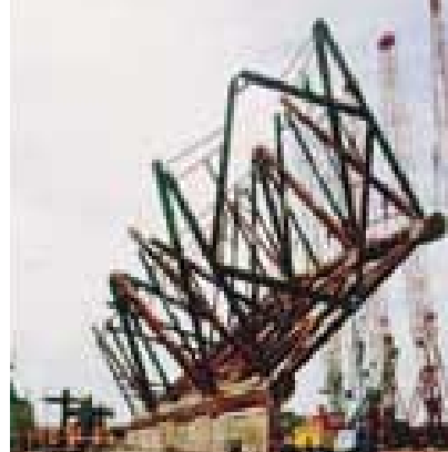
Fabrication of the MIPQ jacket at Sime SembCorp Engineering's Teluk Ramunia yard Fabrikasi jaket MIPQ di kawasan Sime SembCorp Engineering di Teluk Ramunia
